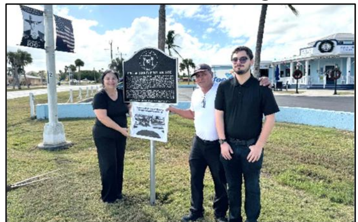
ESHP with the help of Magy, Morgan, and their son Andres, installed the historic Old Jail Site sign in front of Captain Morgan's Seafood Grill near the Circle in Everglades City.
