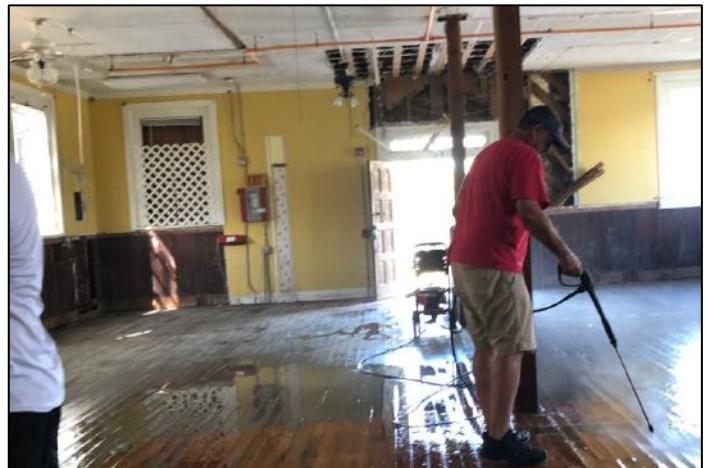
The Bank of Everglades after Hurricane Ian on September 28, 2022.
